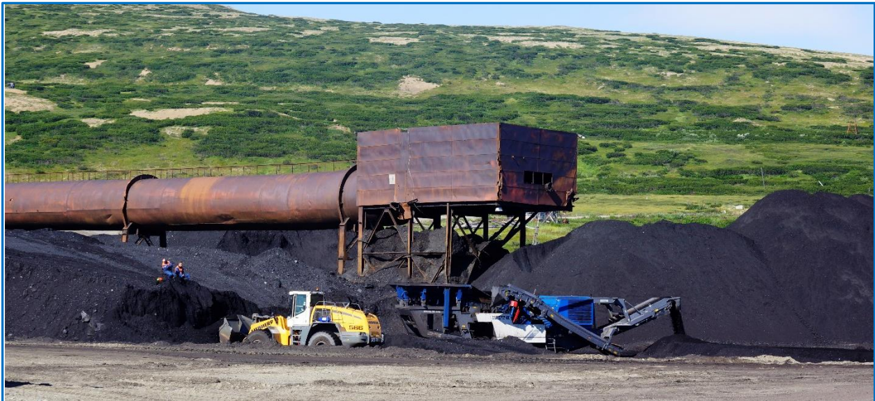
Coal crushing operations at the port stockpiles
