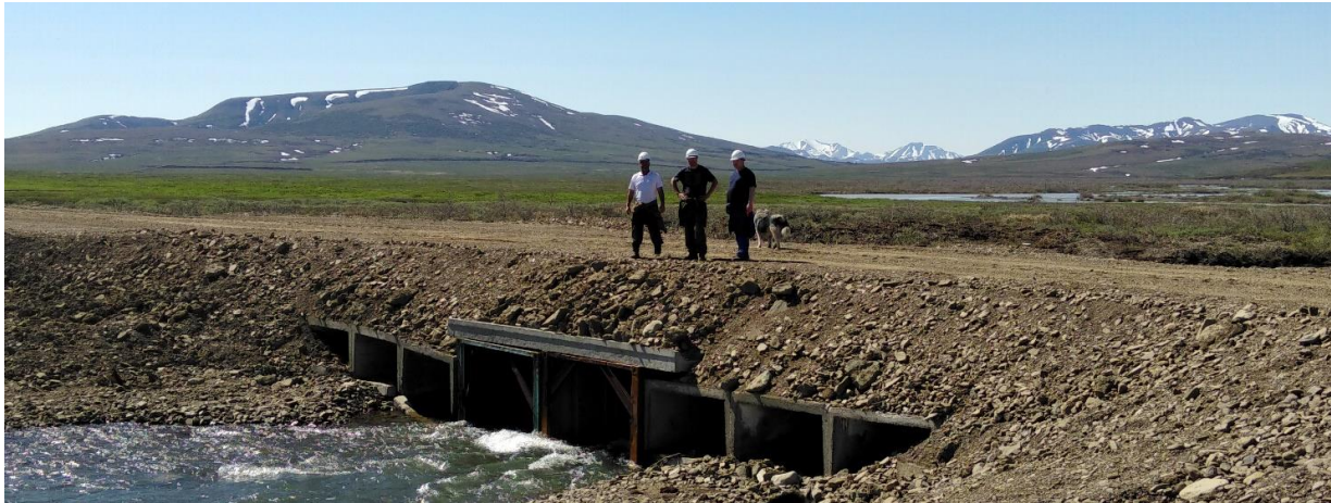
Completed section of road - Marcus Trost (Operations Manager), Anatoly Nikolaev (GM Operations) and Ivan Subbotin (Mining Manager) inspecting a completed river crossing.
